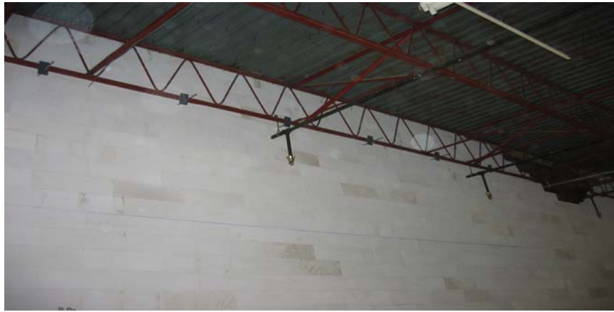
Strip mall renovation using AAC block firewall using melt anchors to attach to bar joist.
