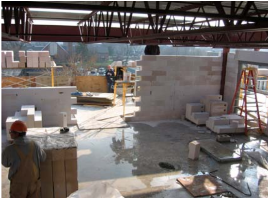
Planning for mechanical opening
